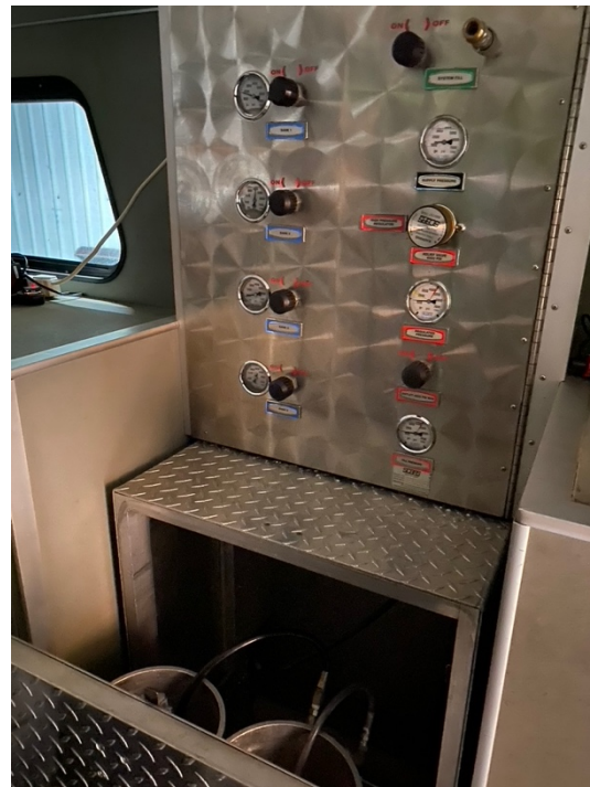
Figure 17 Rescue Truck Air Compressor
